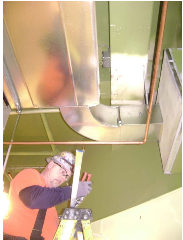
Duct work in Ageless Acupuncture
