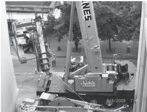
A crane that can lift 550 tons—only two this large exist on the West Coast!—was brought in to lift the Lodril (seen in the upper left) into place.
